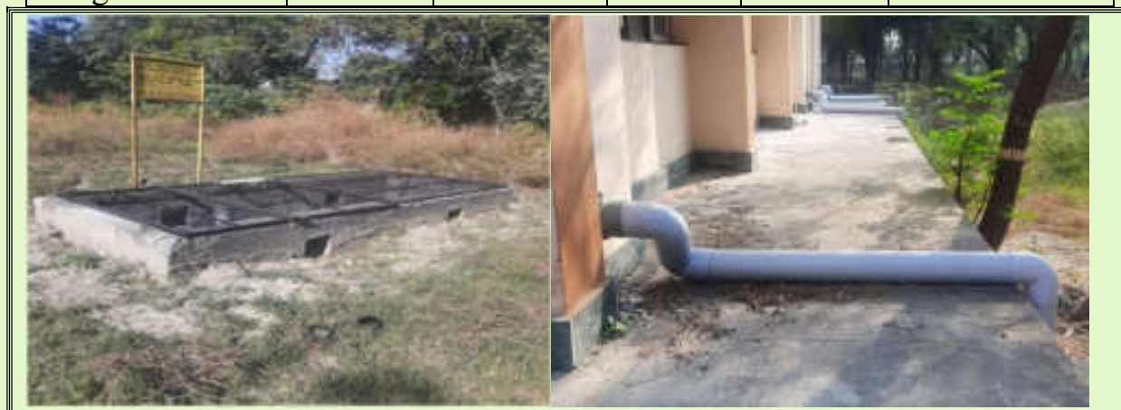
Fig. 2: Rain Water Harvesting Structures installed in the College
