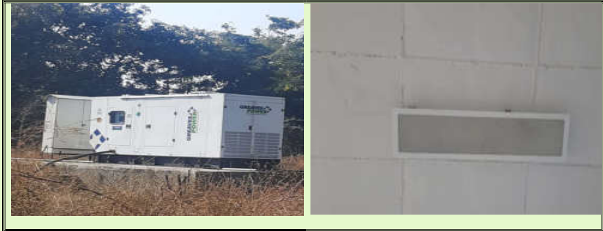
Fig. 3: Energy Saving Installations in the College (32 KVA power substation and LED Lights)
